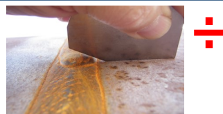
Incorrect angle in connection with the weld run completion
