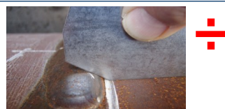
Incorrect angle in connection with the weld run start
